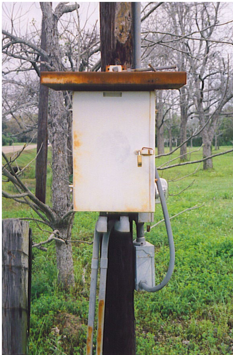
RECTIFIER UNIVERSITY DRIVE (LA. 182)
