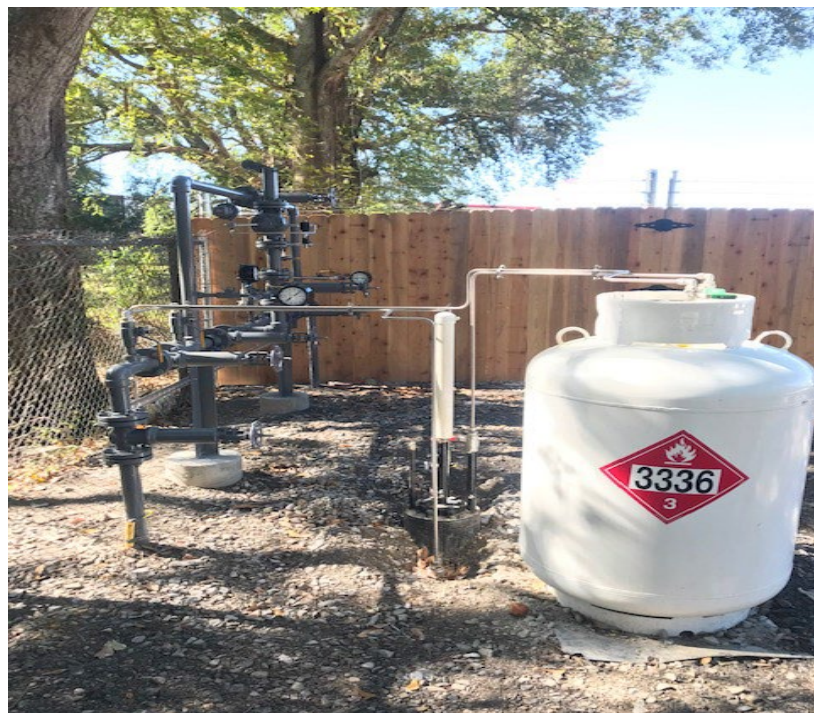
EAST SIDE I-49 REGULATOR STATION
