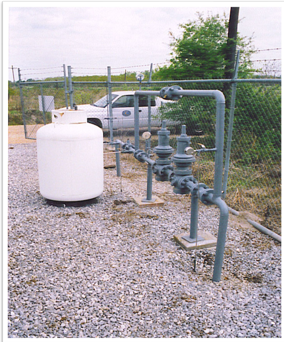
PREJEAN ROAD PURCHASE POINT STATION
